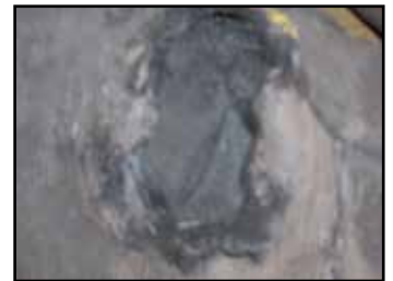
Melted or Charred areas
